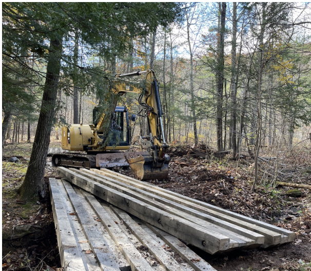
Maintain water quality best management practices for thaw and snow events. (New skidder bridge above)
